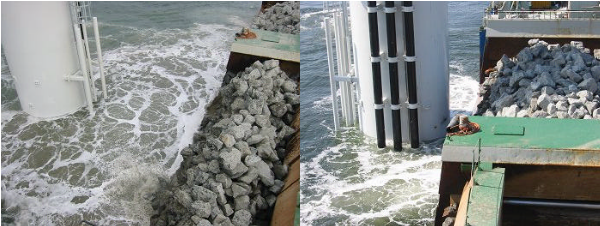
Figure 8 The scour protection was dumped around the foundation. Scour protection are stones ranging from 350 – 550 mm with an average ( d_{50} ) of 400 mm.
