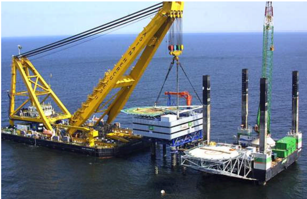
Figure 2 The complete transformer station was lifted onto its 3 supporting piles on 16 April 2002.
