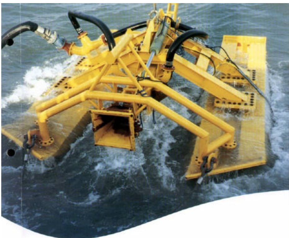
Figure 12 Cables were floated out, connected and finally buried at a minimum depth of 1 m below sea bed by water jetting.
