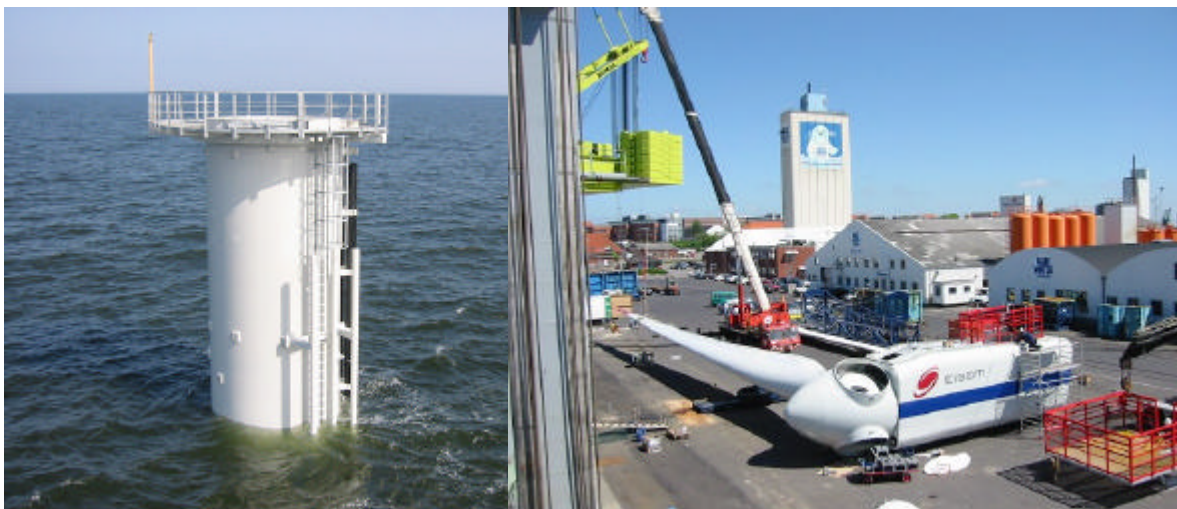
Figure 9 Final installation of platform and J-tubes for cables took place while turbines were pre-assembled and loaded in Esbjerg.
