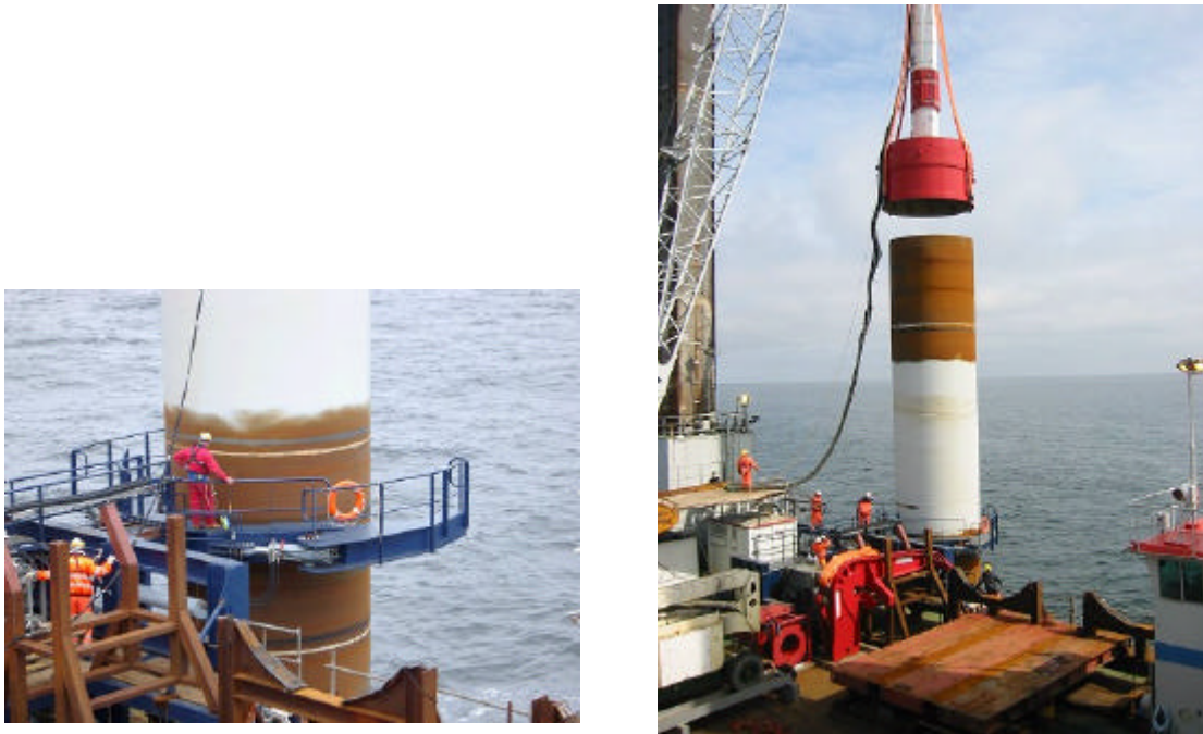
Figure 6 The piles were driven into the sea bed using a 500 t hydraulic hammer. The operation took about 1 hour. Acoustic scaring devices for porpoises and seals were deployed from 1½ hours before start of driving until the end of driving.
